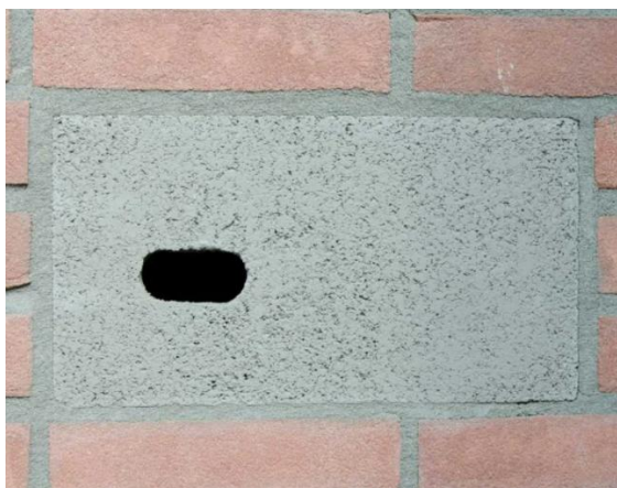
An integrated Swift nesting box in a building
